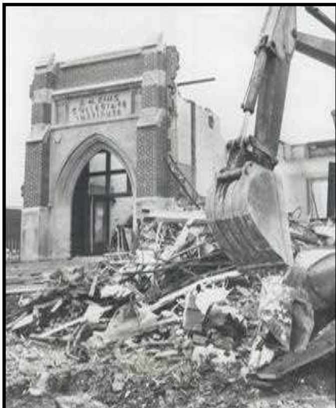
The monumental arches of King have survived both a fire and a demolition.
